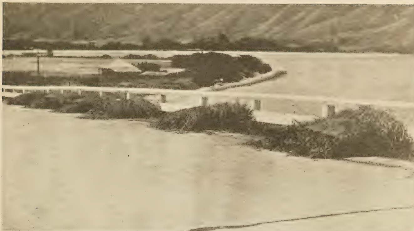
PILES OF WEEDS THAT HAVE FORMED A CARPET OVER THE EDGES OF THE PAVEMENT. THESE WEEDS, ABOUT 6 MONTHS OLD HAVE BEEN CUT AT INTERVALS OF 10 OR 15 FEET AND ROLLED UP PREPARATORY TO REMOVAL.
